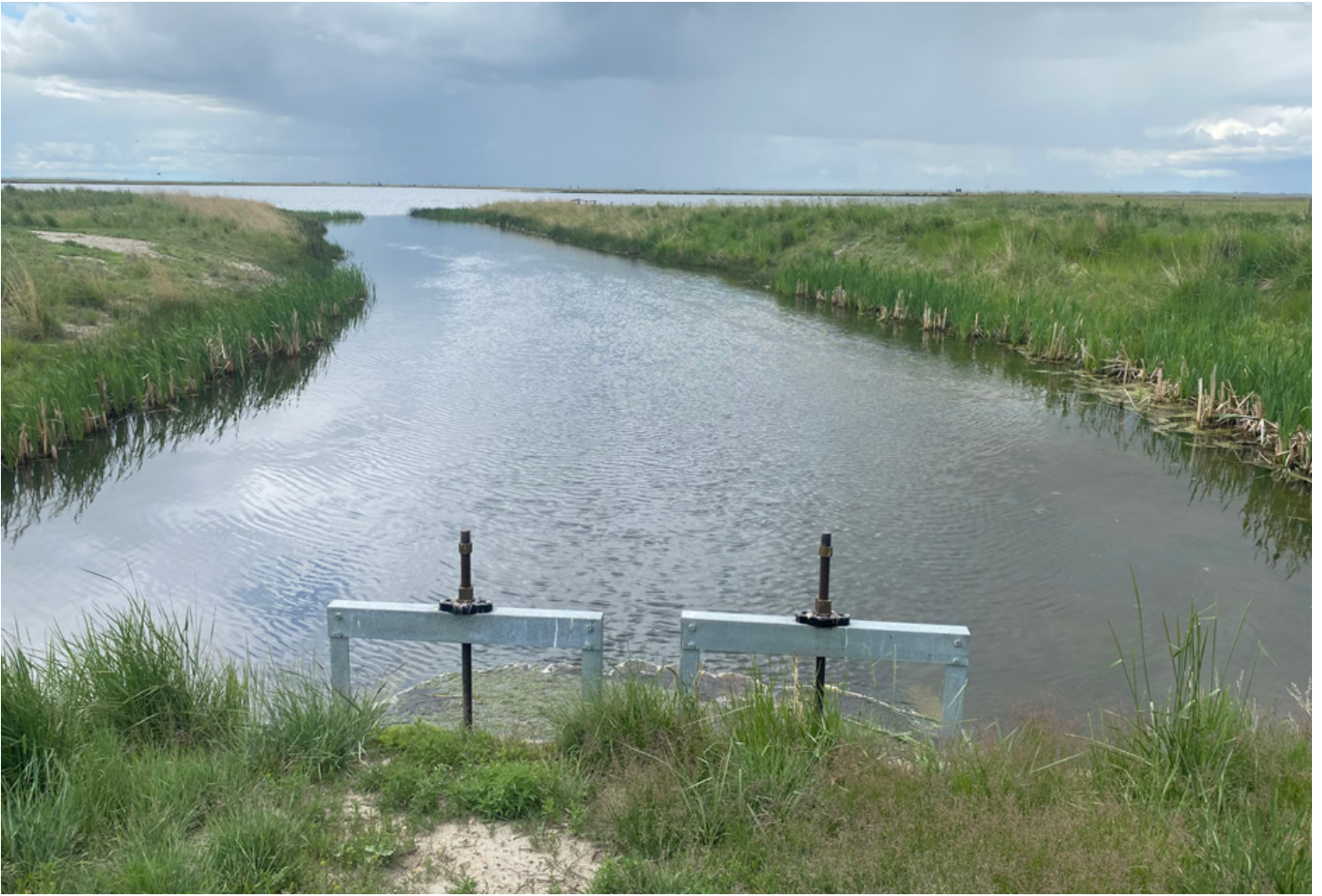
This new structure at Crab Lake was funded by Pheasants Forever Calgary two years ago, and guarantees water delivery to several wetlands across the EID North Pastures.
